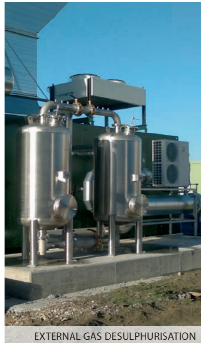
EXTERNAL GAS DESULPHURISATION
