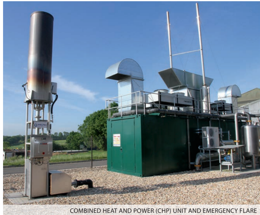
COMBINED HEAT AND POWER (CHP) UNIT AND EMERGENCY FLARE
